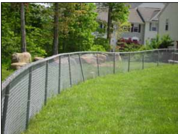
Photo #5. Minor damage to the outfield fence at the ball field.
