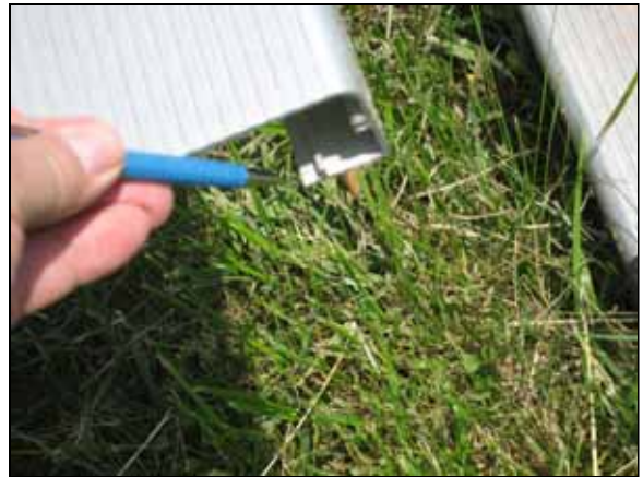
Photo #4. Missing end cap exposes a sharp edge, bleachers at ball field.
