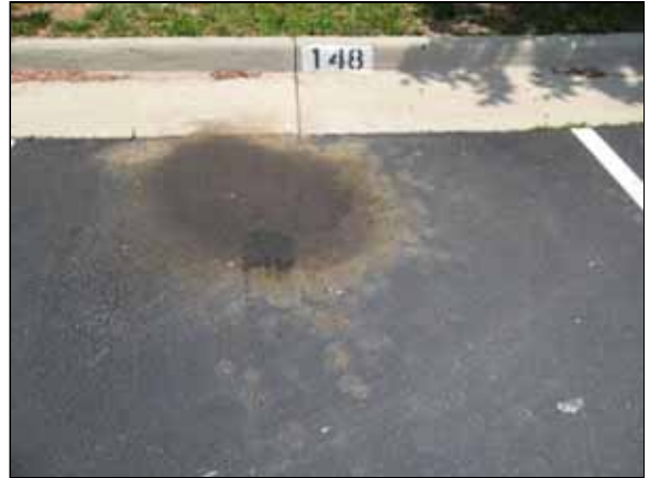
Photo #14. Asphalt pavement damaged by oil/gasoline, Penny Tree Place.
