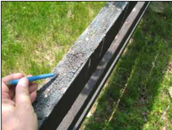
Photo #39. Deteriorated paint on the three rail wood fence at the entrance feature.
