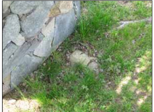
Photo #38. Grading at the entrance feature impounds water against the entrance feature.
