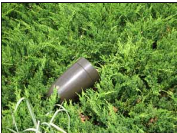
Photo #41. Ground mount light fixture at the entrance feature.
