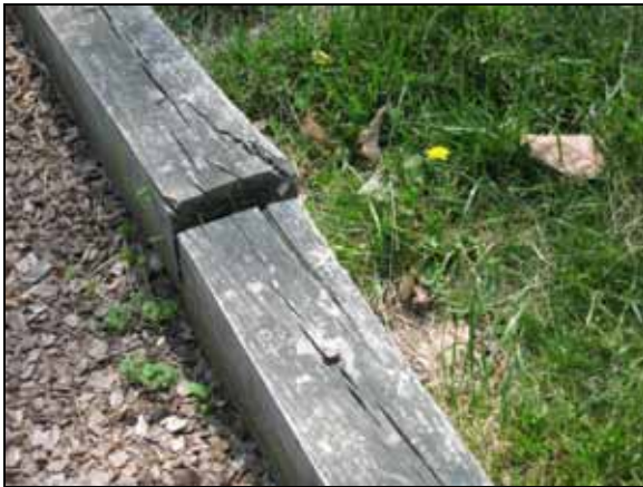
Photo #27. Deteriorated tot lot wood border, Gaston Tot Lot.
