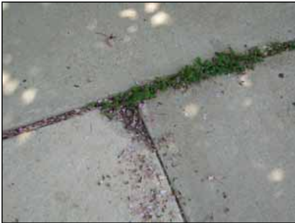
Photo #15. Typical minor defect in the concrete sidewalk, 4563 Penny Tree Place.
