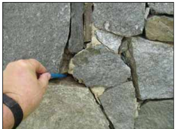
Photo #36. Minor defects in the entrance feature.
