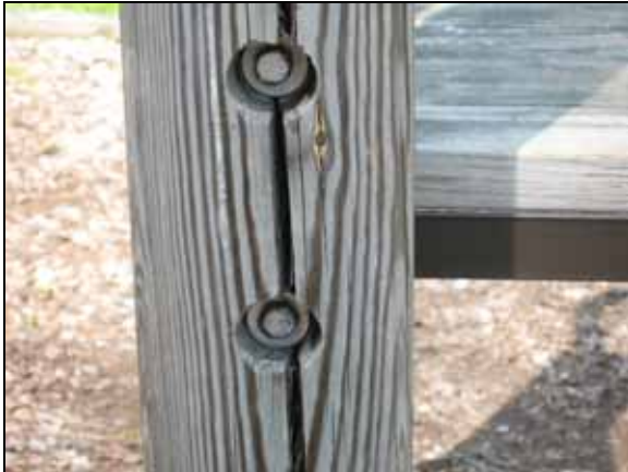
Photo #31. Severe checking of support post, Gaston Tot Lot.
