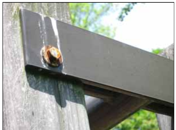
Photo #30. Deteriorated fastener, Gaston Tot Lot.
