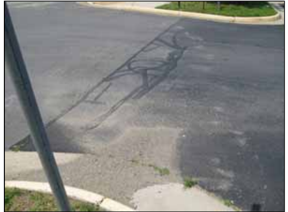
Photo #20. Deteriorated asphalt pavement and depressed curb & gutter segment at the intersection of Penny Tree Place and Eagle Chase Circle.
