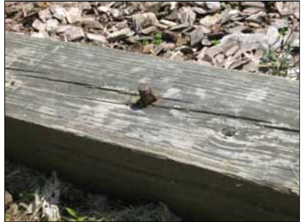
Photo #26. Rebar used to install the border at the Gaston Tot Lot is a potential trip hazard.
