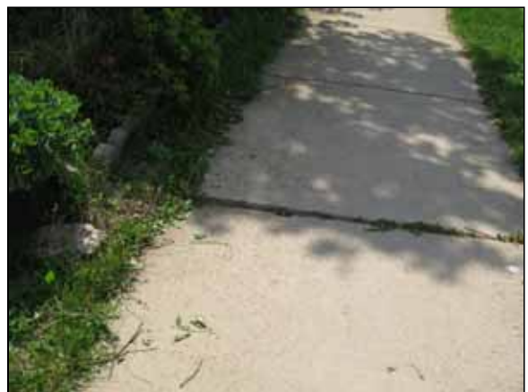
Photo #12. Typical minor displacement of concrete sidewalk, 4559 Penny Tree Place.
