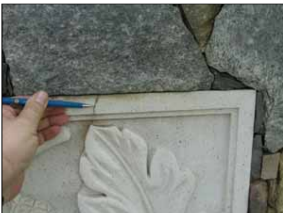
Photo #35. Cracking of precast components in the entrance feature, Eagle Chase Road and Walney Road.
