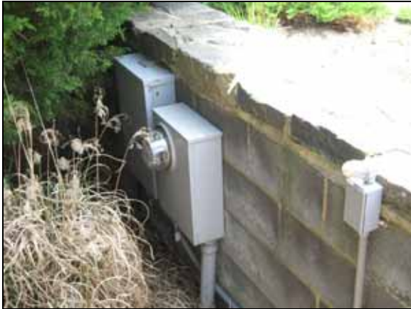
Photo #43. Common electrical service installed at the entrance feature.
