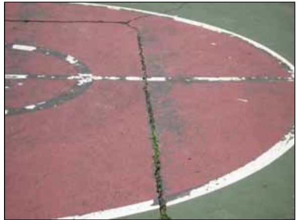
Photo #10. Failed color coat and large open cracks in the MP court.
