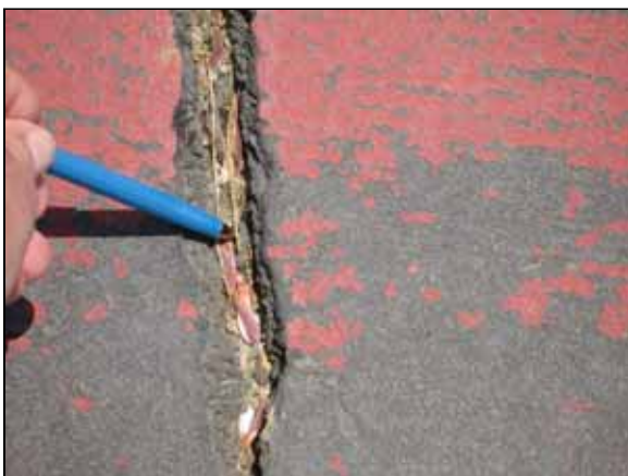
Photo #11. Failed color coat and large open cracks in the MP court.
