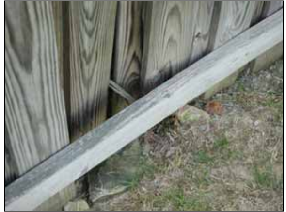
Photo #46. Defect in the stockade fence installed along Walney Road.
