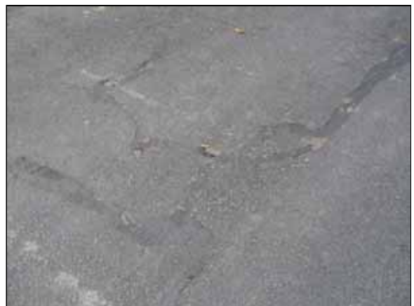
Photo #18. Cracking of asphalt pavement, Penny Tree Place.
