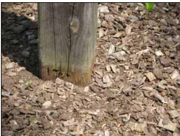
Photo #29. Deteriorated wood post, Gaston Tot Lot.
