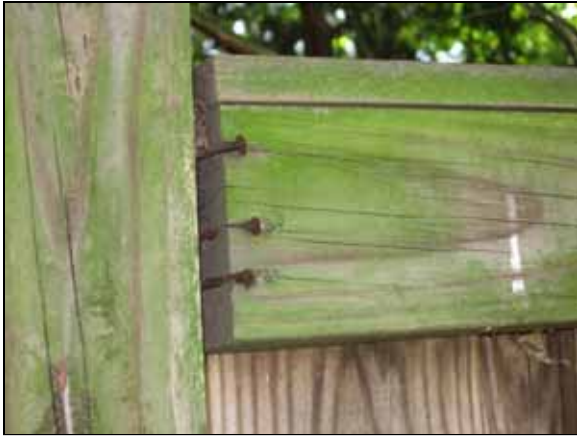
Photo #45. Defect in the stockade fence installed along Walney Road. Note organic growth.
