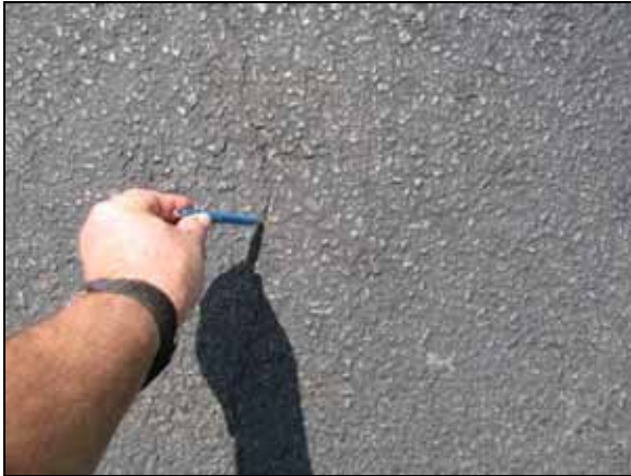
Photo #13. Minor cracking the asphalt pavement that should be crack sealed, Penny Tree Place.
